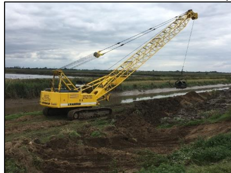
De-silting of the tidal River Nene, on behalf of the EA, by North Level District IDB
