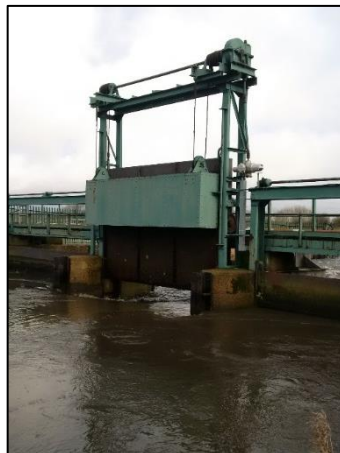
Stanground Sluice in operation
